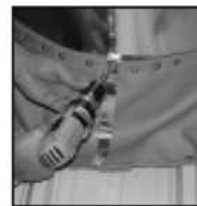
5. Fasten through top of termination strip, Dekstrip, and back of strip with Scotfasteners or rivets.
